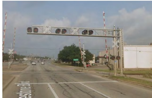
Figure 4: Existing overhead RR crossing structure at Red Line and E Whitestone Blvd (Source: Google Maps)
